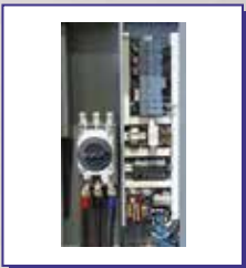
Control panel and circuit breaker
